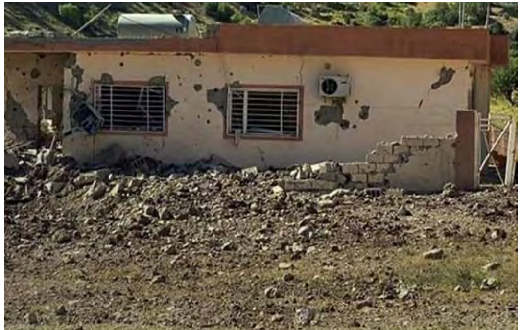
A residence in the Kurdistan Region that was damaged by recent Turkish airstrikes targeting alleged Kurdistan Workers' Party (PKK) positions, May 27, 2020. (Photo: Kurdistan 24)
