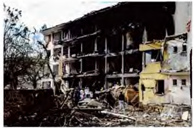
A building in Diyarbakir that was damaged by a car bomb in January 2016. Credit Ilyas Akengin/Agence France-Presse — Getty Images
